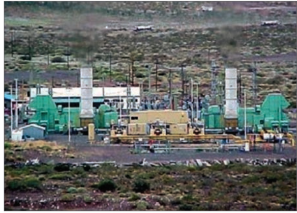
Figure 12 – 2 X LM2500 power plant operating on lean methane fuel.
