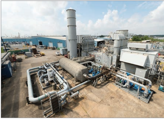
Figure 11 – GE aeroderivative gas turbine test facility.
