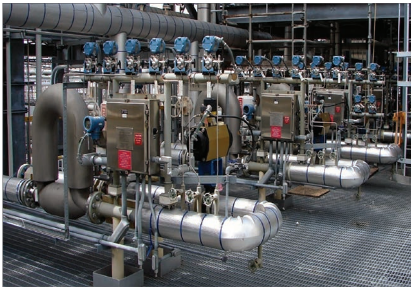
Figure 14 – Fuel blending systems for multiple F-class gas turbines.
