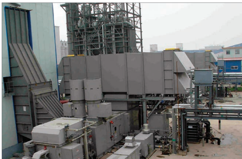
Figure 10 – LM2500 gas turbine generating power from COG at a steel mill plant in China.
